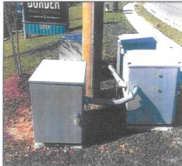
"New wood pole (holding up cell and microwave antennas) and equipment enclosures for a 'Small Cell' (appears to be by 'Mobilitie' for Sprint) in the public right of way (where all other . . . utilities are already underground) in Woodbridge, Virginia."
